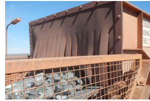
Enclosure of dusty machines & transfer points
