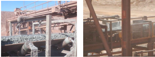
Use of dust suppressant chemicals & water sprays at transfer points
